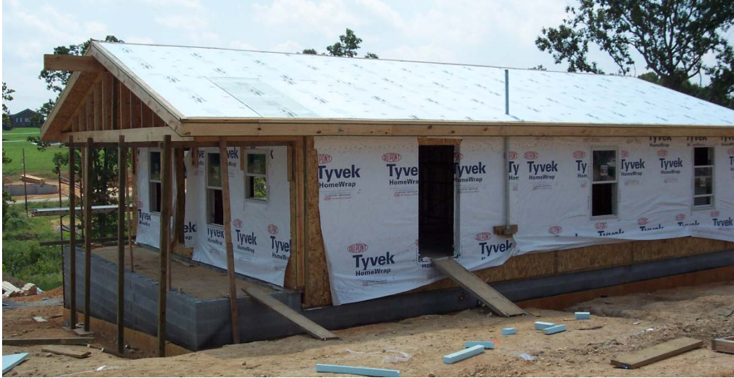
Fig. 5. Before the metal roofing is installed, 2 in. of XPS is laid directly on top of the 8 in. thick SIP roof panels.
