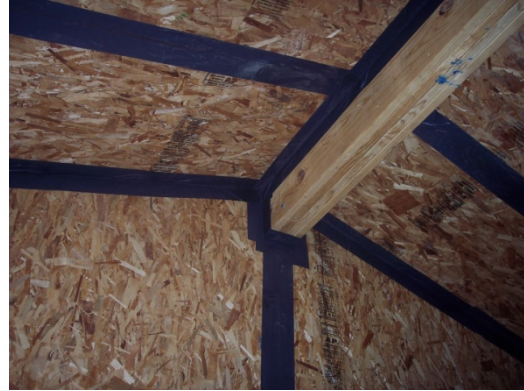
Fig. 27. Peel-and-stick panel tape provides added assurance that panel seams will remain airtight.
