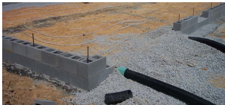
Fig. 26. Footer drains run to daylight on both sides of the wall below the walkout lower level floor.
