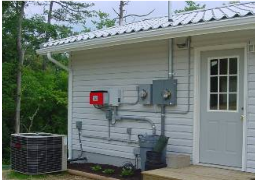
Fig. 51. Sunny Boy (red box at left) installed in TVA-approved Green Power Generation hookup.
