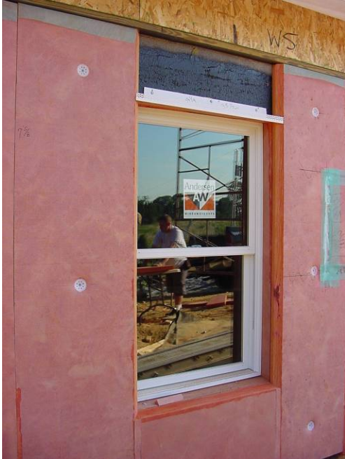
Fig. 24. Detailing around inset windows to avoid thermal shorts and minimize water penetrations is very important.
