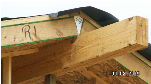
Fig. 43. A wedge of foam is provided by the SIP manufacturer to fill the space at the ridge.
