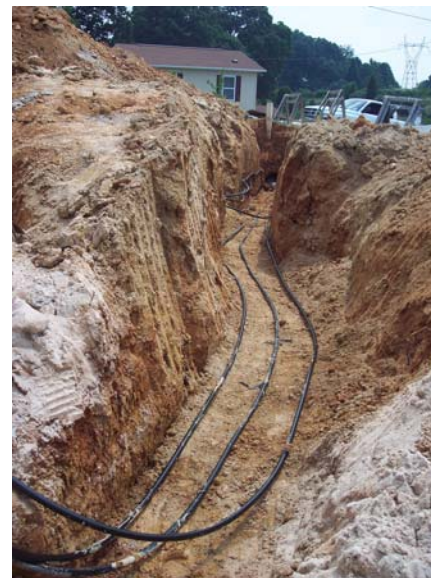
Fig. 35. Ground loop being installed in the bottom of the sewer pipe trench.
