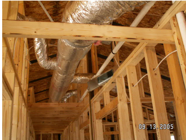
Fig. 37. Supply ducts located in the conditioned chase formed by the ceiling SIP and dropped ceiling.
