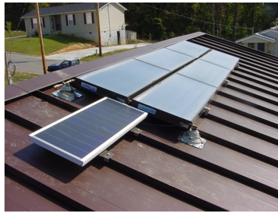
Fig. 6. Solar water heater collectors and the 11 W PV panel to power a 12 V DC pump.
