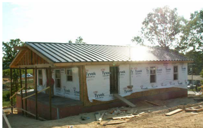
Fig. 31. Infrared selective coating was used on the brown raised metal seam roof to cover ZEH5.
