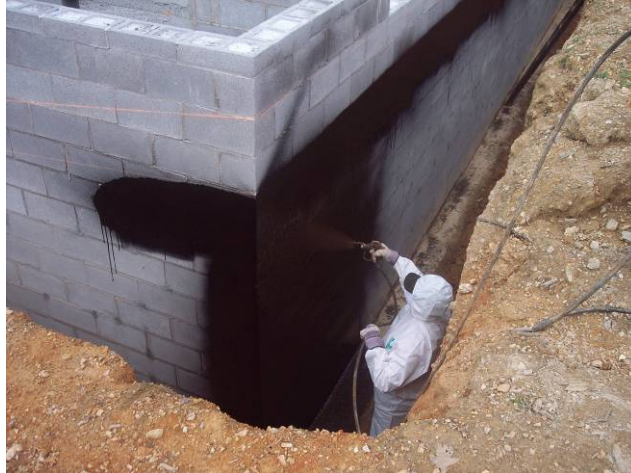
Fig. 22. Waterproofing. For OSHA compliance, the over cut of the house must be sloped 45° for depths greater than 5 ft.
