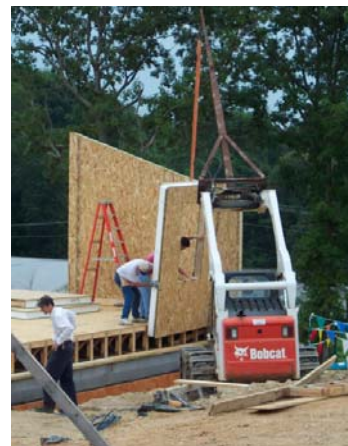
Fig. 44. Mounting the wall panels on the side of the floor trusses leaves easy access to run electric wires from the walkout lower level into the vertical wiring chases in the wall SIP.
