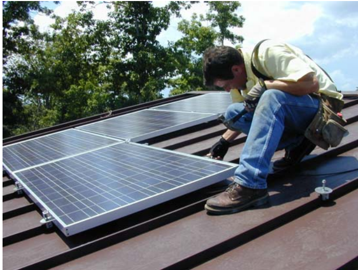
Fig. 48. Solar modules on the roof of ZEH5 are installed directly to the raised metal seam using the S5 mini clamps without the rails typically run parallel to the raised seams.
