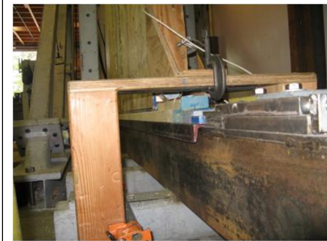
Figure E3. Bottom plate detail, the 4-1/2" wide SIP wall sitting on top of a 2x6.
