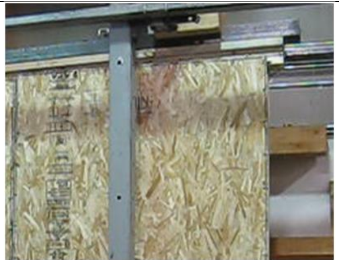
Figure E4. Typical ultimate failure mode of top plate coming unattached to wall studs.
