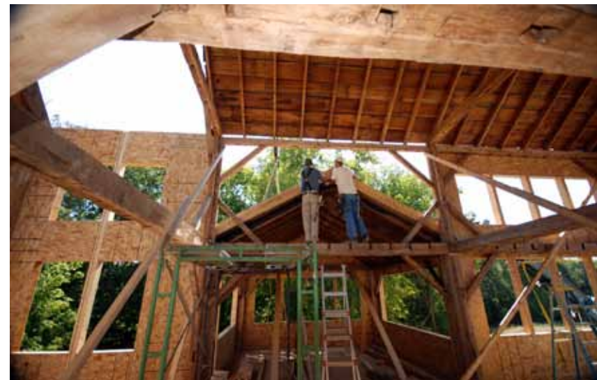
(Above) The original 1862 farmhouse during disassembly. (Below) Crews enclose the salvaged timber frame with structural insulated panels.
