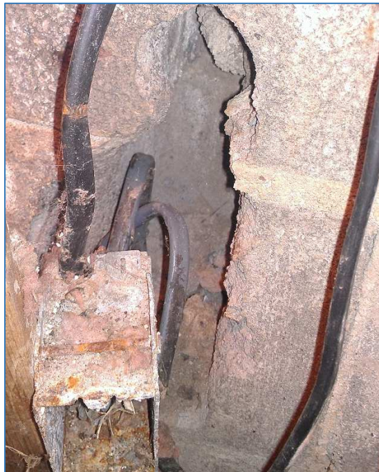
Figure 22. Abandoned Basement Receptacle at CMU Wall
