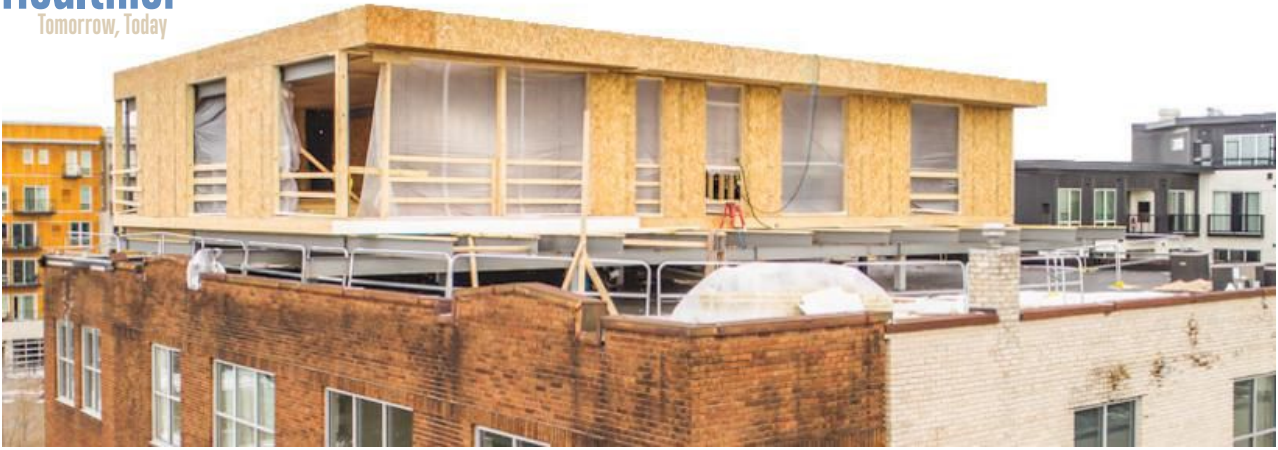
The 3,410 square foot Bryant Residential Loft was a fourth-level to an existing three-story masonry building, and SIPs were able to help reduce crane time and labor compared with the costs of conventional framing and insulation. Credit: Courtesy of Energy Panel Structures
