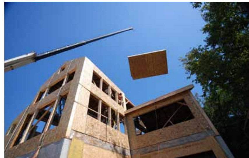
(Above) A large section of SIP wall panels is preassembled on the ground and lifted into place. (Below) Eight-inch-thick SIP roof panels complete the energy-efficient building envelope.
