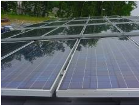
Figure 46. PV modules are clamped to aluminum rails and carefully grounded.
