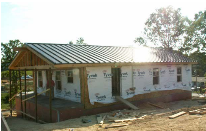
Figure 30. Infrared selective coating was used on the brown raised metal roof to cover ZEH5.
