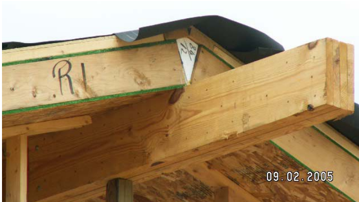
Figure 41. A wedge of foam is provided by the SIP manufacturer to fill the space at the ridge.
