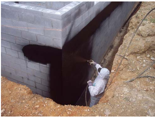
Figure 21. Waterproofing. Note to be OSHA compliant the over cut of the house needs to be sloped 45° for depths greater than 5 ft deep.
