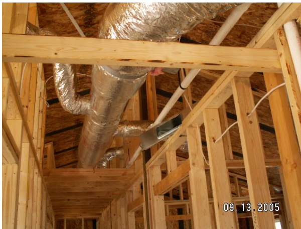
Figure 36. Supply ducts located in the conditioned chase formed by the ceiling SIPS and dropped ceiling.
