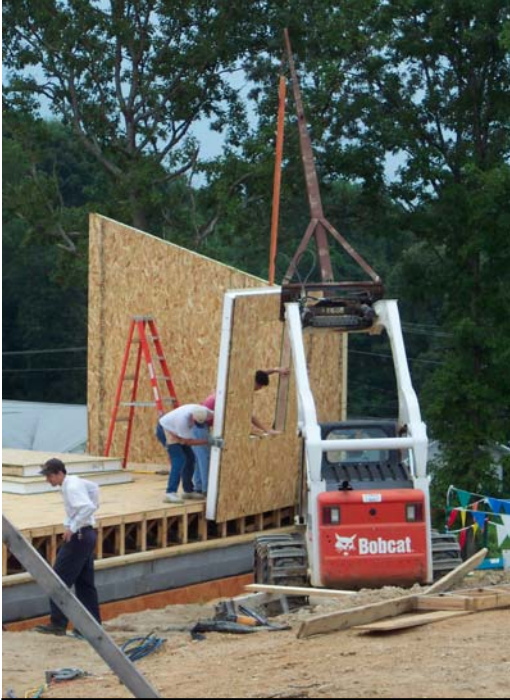
Figure 42. Mounting the wall panels on the side of the floor trusses leaves easy access to run electric wires from the basement into the vertical wiring chases in the wall SIPs.
