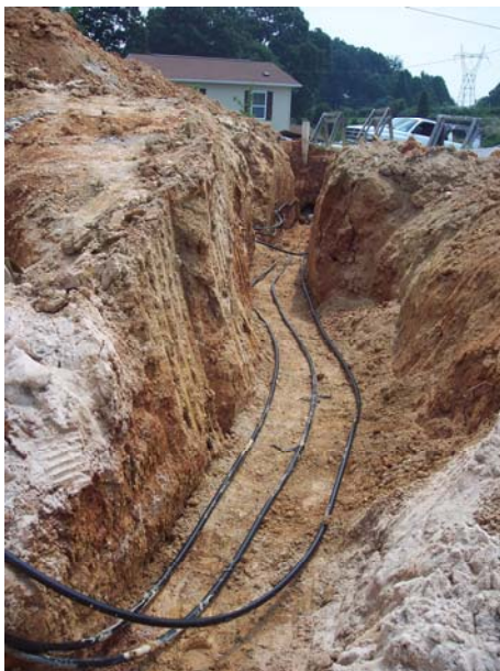
Figure 34. Geothermal heat exchanger pipe being installed in the trench dug for sewer lines.
