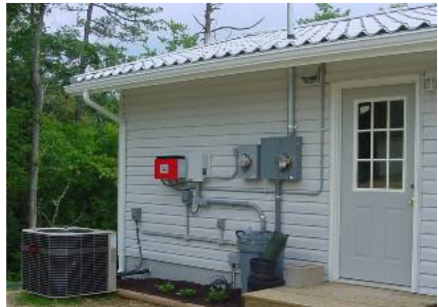
Figure 48. Sunny Boy (red box at left) installed in TVA-approved Green Power Generation hookup.
