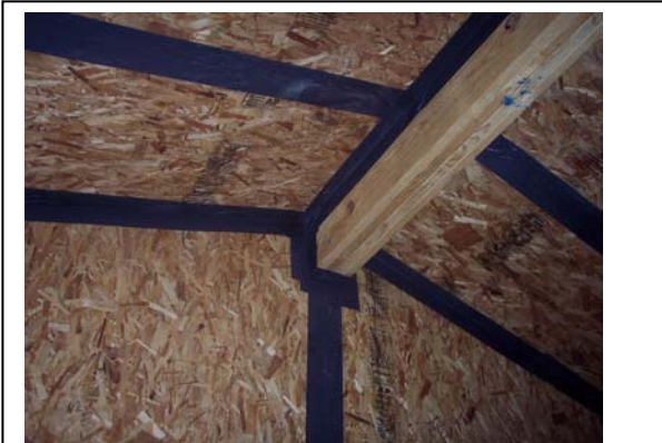
Figure 26. Peel-and-stick panel tape provides added assurance that panel seams will remain airtight.
