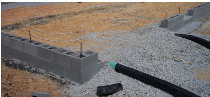
Figure 25. Footer drains run to daylight on both sides of the wall below the basement floor.
