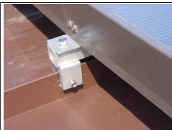
Figure 31. S-5 mini clip holding a solar module on ZEH5 to the raised metal seam.
